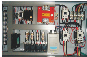
AC電氣箱 AC Electric Box
